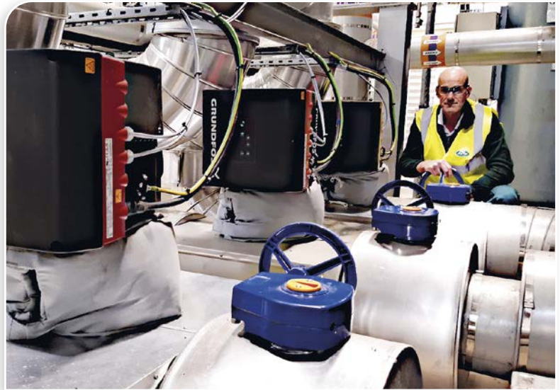
George Nicholls, Arla Foods, and the new TPE pumps for the ice water system (photo: Grundfos)
