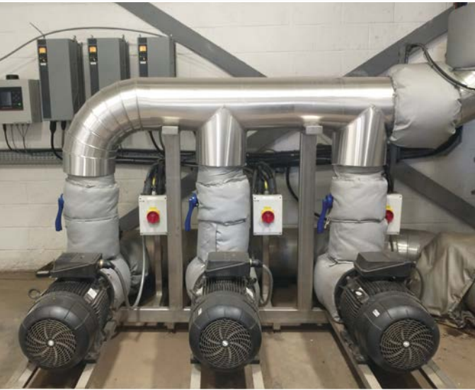
The new chilled water NB pumps at Arla's Westbury dairy (photo: Grundfos)
