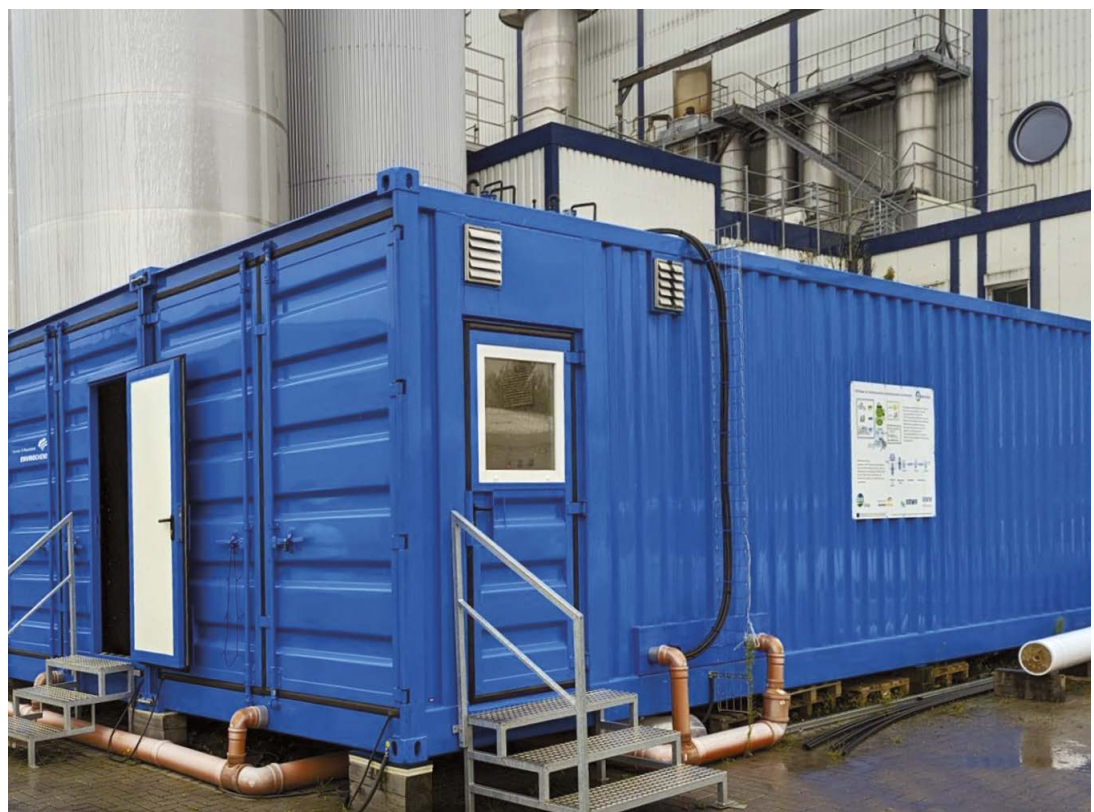
Test plant housed in two containers for processing evaporator condensate into drinking water (photo: IDM)
