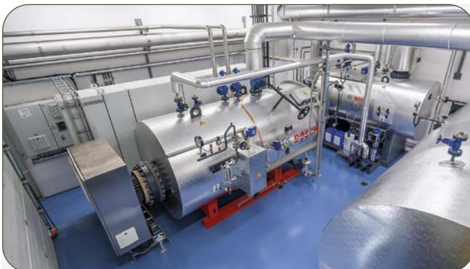
Electric steam boiler system from Bosch with 100 per cent green power utilisation (photo: Bosch Industriekessel)
