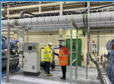
Existing refrigeration plant room at Britvic with three GEA BluAstrum chillers. Their waste heat will also feed the new heat pumps (photo: GEA)
