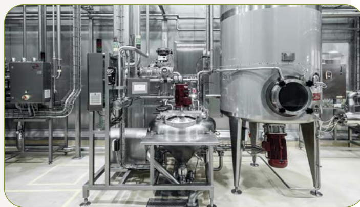
Mixing plants and syrup rooms lay the foundations for the quality of the end product (photo: Ruland)
